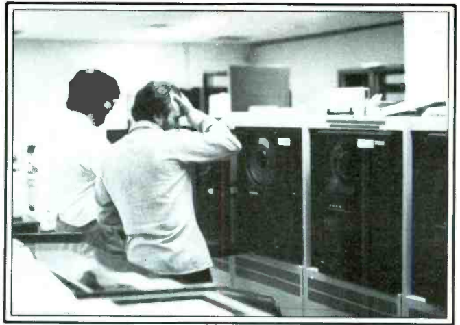
Instead of loudspeakers for listening, tape recorders in the Control Center record the noise of radio sources received from antennas through an underground waveguide.
